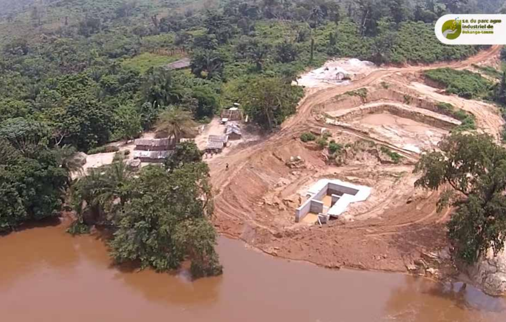
Pumping station for the irrigation of the Bukanga Lonzo agro-industrial park in DRC, source: http://www.parcagro.com/
