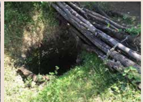
A bundle of wood placed across an old destructed well to prevent people from falling
